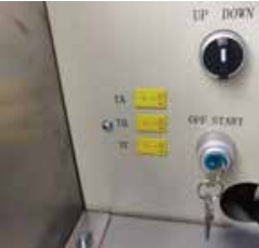
▲ 温度曲线测试接口 Temperature curve test interface
