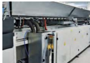
Maintenance "On-the-Fly" continues to operate while the condensation management system is being cleaned
