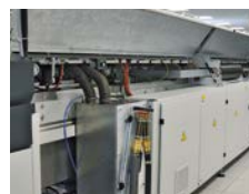
Maintenance "On-the-Fly" continues to operate while the condensation management system is being cleaned
