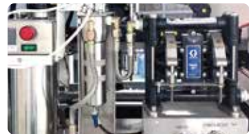
Closed loop fluid heating system
